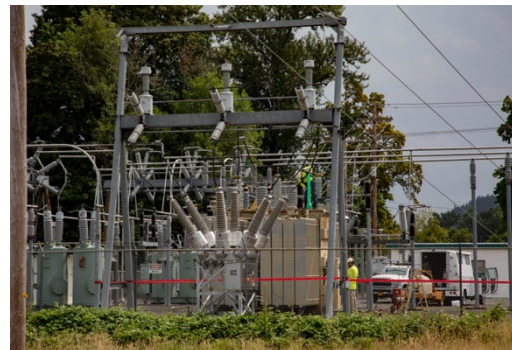
EWEB’s High Banks Substation
